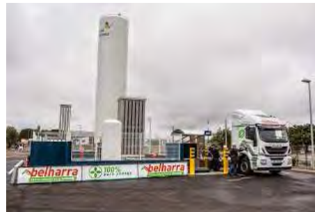
Station GNL/C de Castets GAS NATURAL FENOSA
